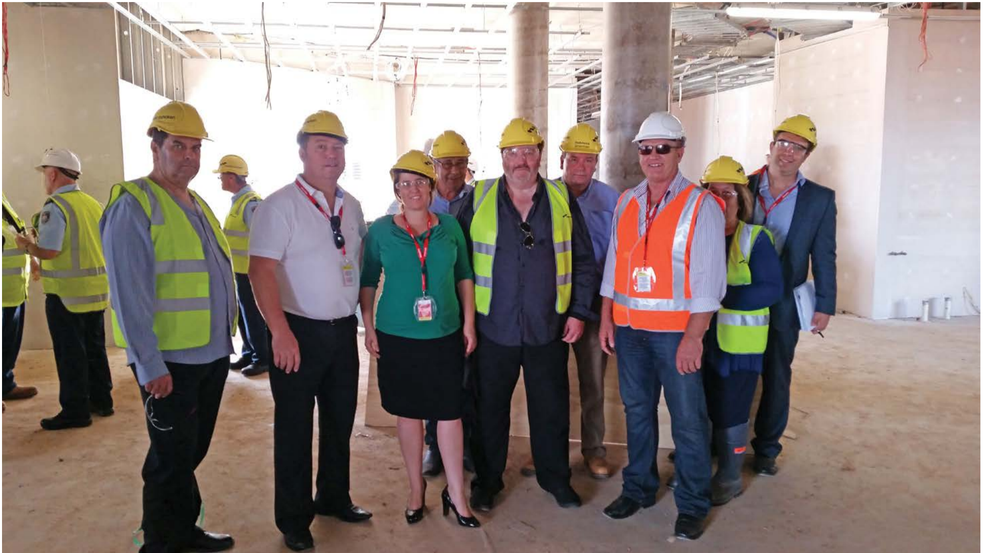
The new facility is undergoing construction. PSA representatives inspect the site. Left to right: COVB representative Darren Wells, PSA General Secretary Stewart Little, PSA President Kylie McKelvie, COVB representative Mark Christensen, COVB Chair Greg Delprado, Central West non-custodial representative Scott Chapman, POVB Industrial Officer David McCauley, COVB representative Janet Beer, PSA Manager Industrial Specialist Shay Deguara.
